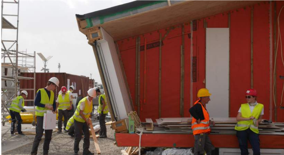
Photo 3- Virtue-Netherlands- University of Eindhoven. This part represents an unachieved apartment next to the real prototype (behind) as if it was on a collective building. Credit FYusta
