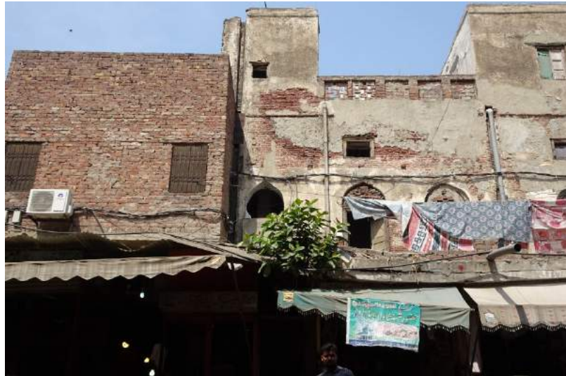
Figure 1. Split air conditioner fitted to uninsulated brick building in Lahore (2016: outdoor unit can be seen at far left side)
