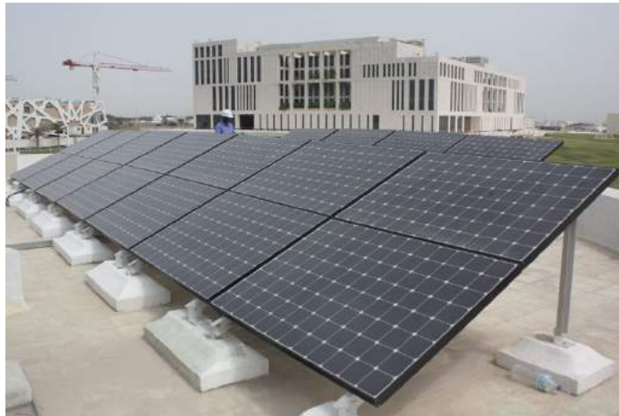
Figure 2. The roof-mounted PV system with ballasted racking
