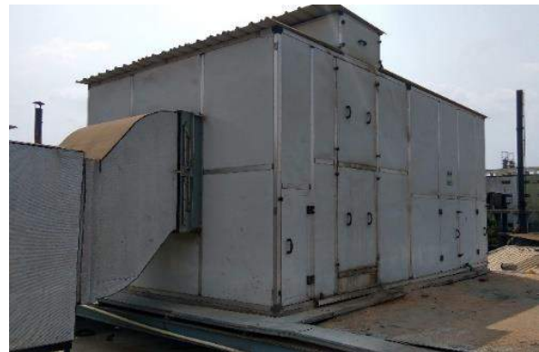
Figure 4: IDEC as installed on site
