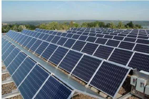
Figure 2. The PV cells, source: https://encrypted-tbn0.gstatic.com
