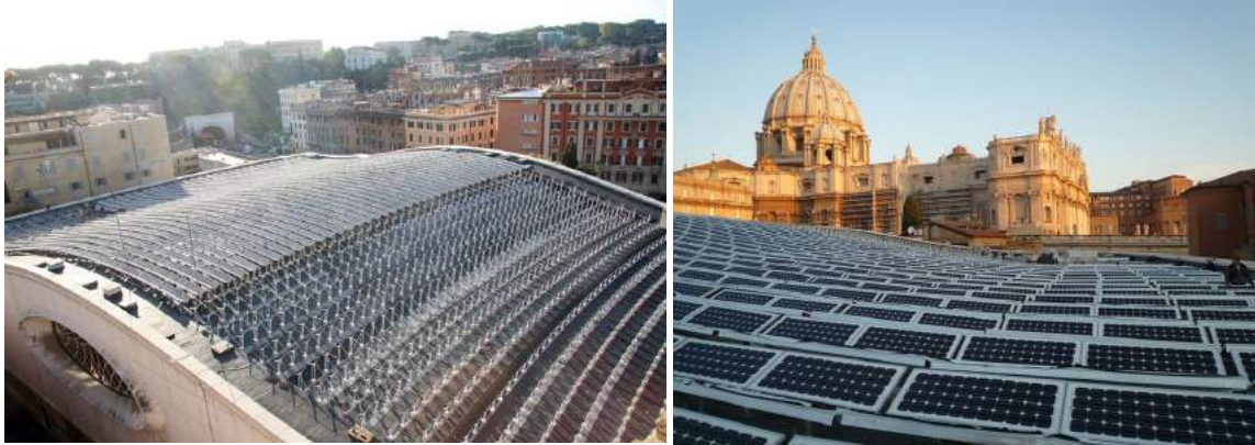
Figure 3. Photovoltaics panel on the roof of the historic Paul VI Audience Hall in Italy https://www.archilovers.com/projects/14001/copertura-solare-dell-aula-paolo-vi-in-vaticano.html#images
